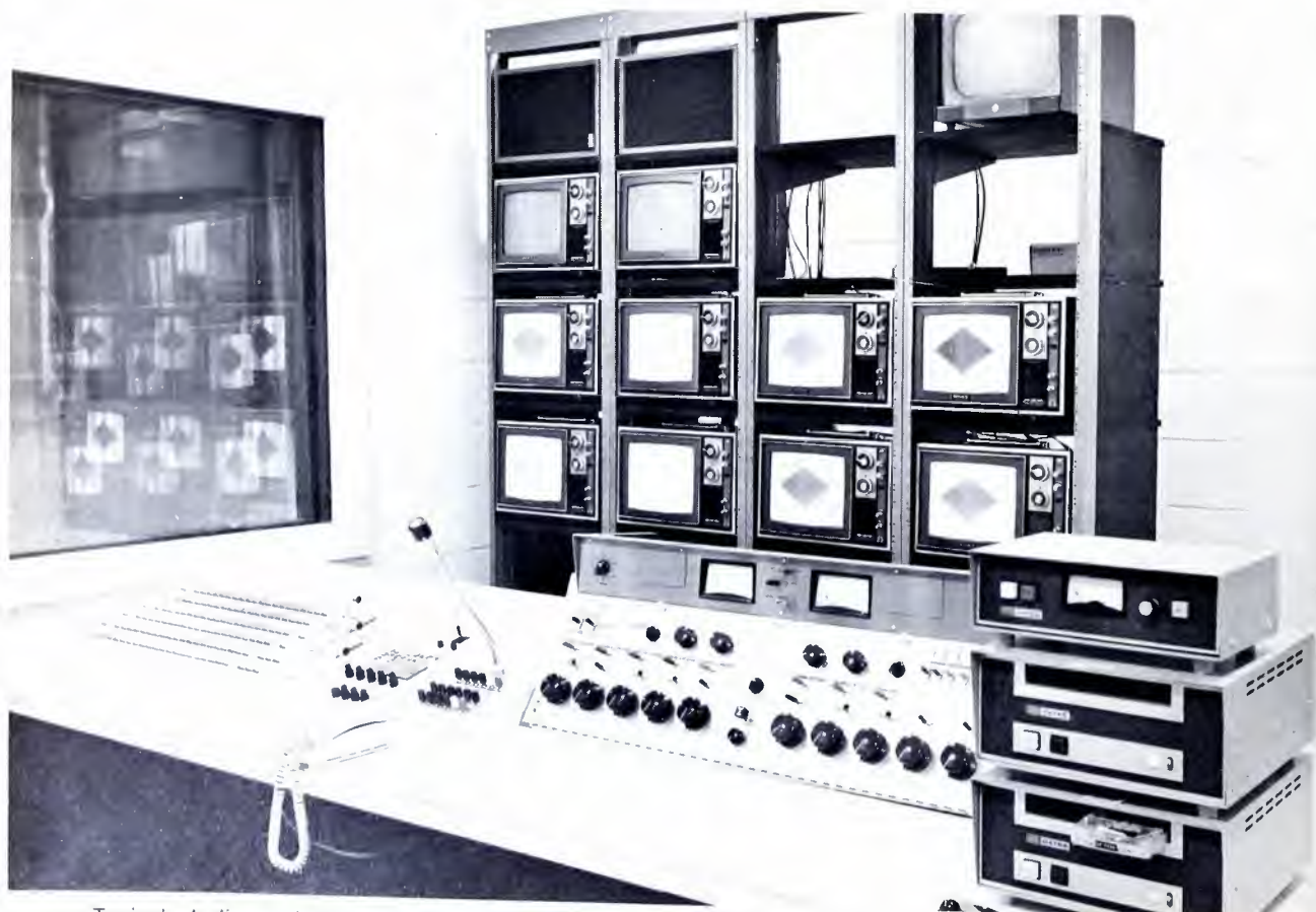
Typical studio control room showing new Grass Valley switcher, RCA audio console, and Gates cartridge tape equipment. Monitors are "jeeped" Sony 1201 color receivers.
