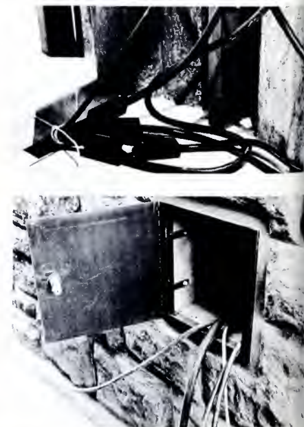
(Top) Cableraceways at all conceivable camera positions keep cable from being exposed to view. (Bottom) The mobile unit can be hooked up to the sound system in the cathedral from the outside, eliminating the laying of cables.
